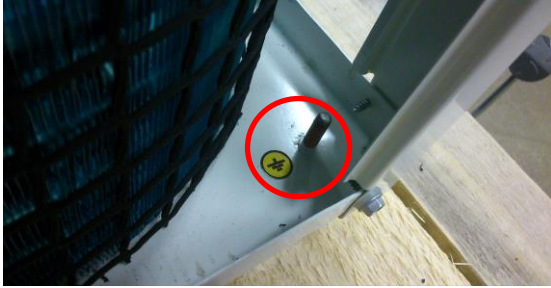
Figure 9: Additional ground connection on the unit baseplate
