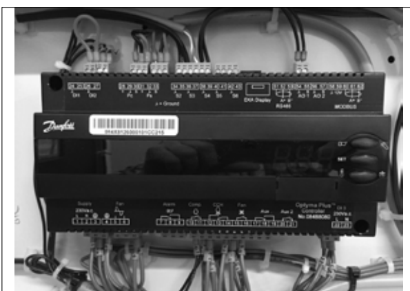
Picture 4 : Normal wiring
