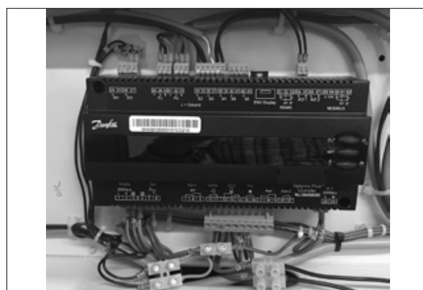
Picture 5 : Temporary wiring
